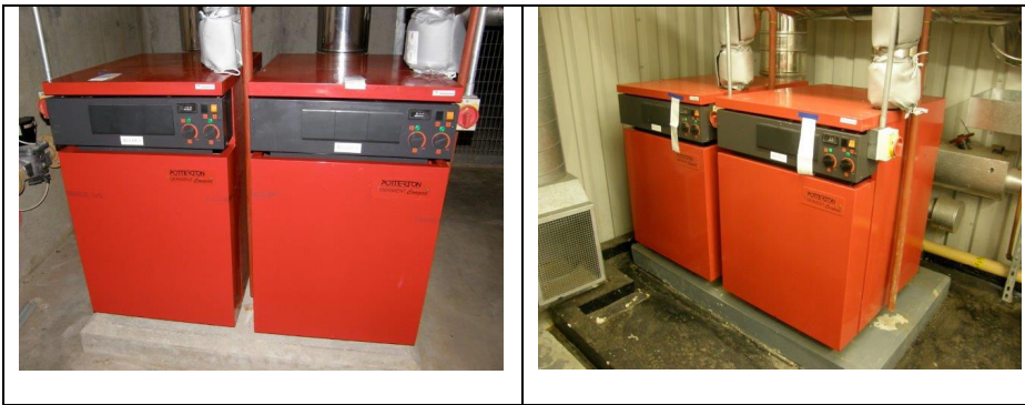
Image a. Capswood 1 underground. Image b. Capswood 2 Roof plant room
